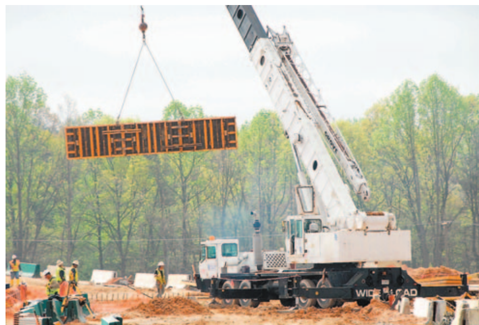
Construction workers place forms for the grade beams at the central utility plant building.
