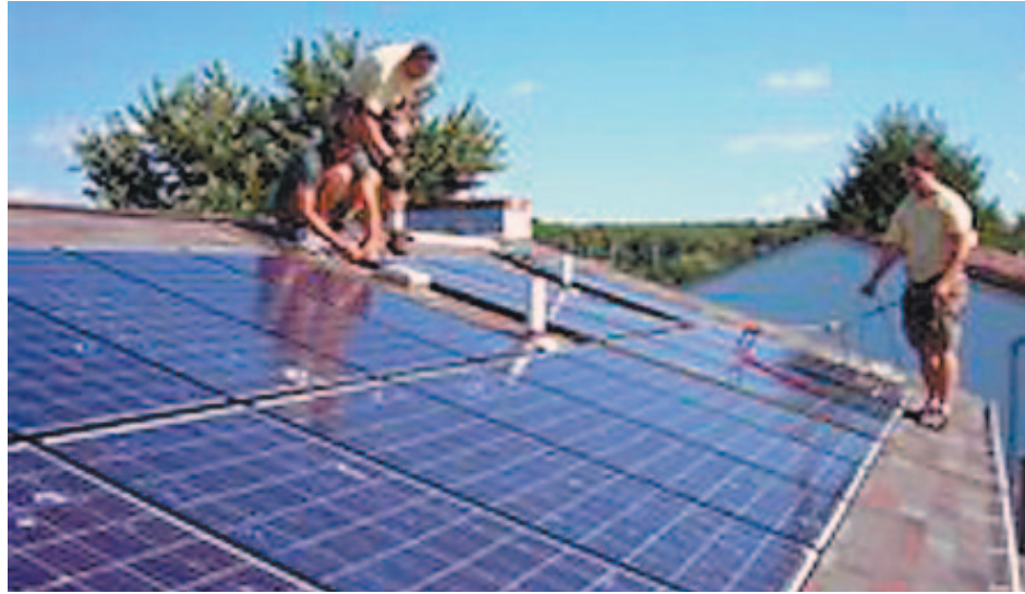
The hardest part of getting solar panels was deciding what to get and figuring out how to get it, Richard Watts said. The actual installation, shown here, took a day.
