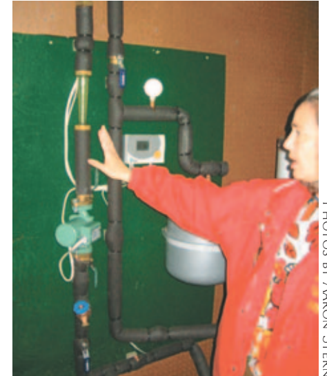
Monique Hanis points out the hot water plumbing.
