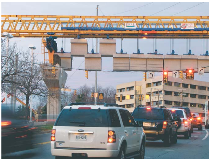
A view of the construction site at the Route 7/Spring Hill Road intersection.
