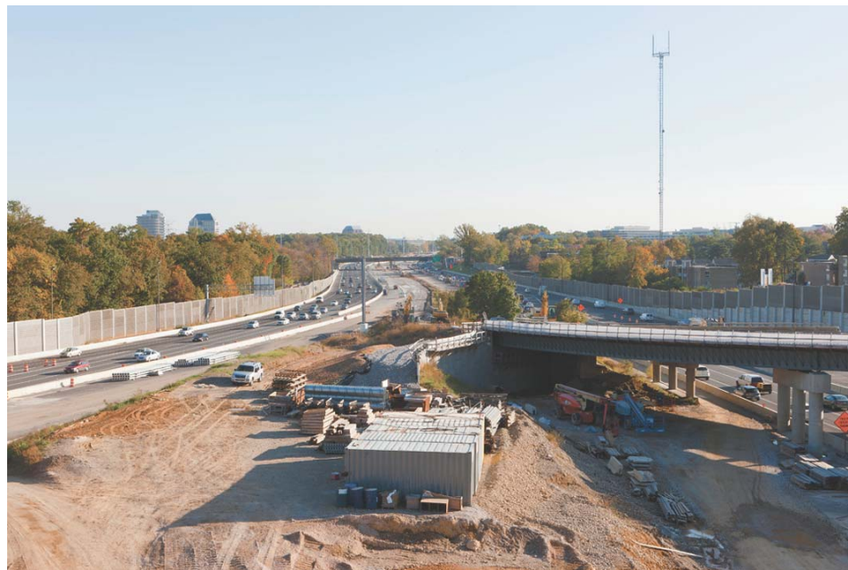
Looking south from the I-66 ramp, the HOT Lanes configuration takes shape.
