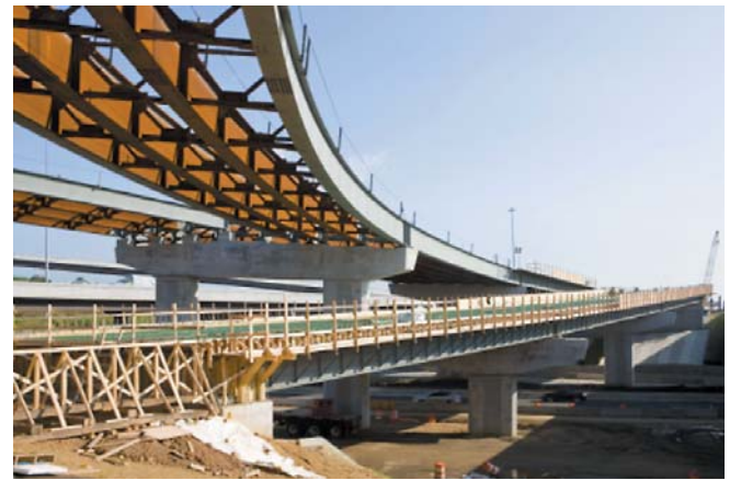
New bridge piers are under development to support completion of project construction in the Springfield Interchange.
