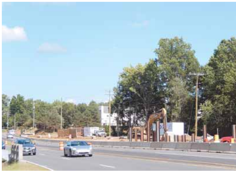
Drivers heading toward Centreville pass the construction site on Route 29 near Union Mill Road.
