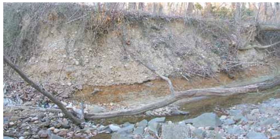
Severe erosion on the banks of Quander Brook below the storm water outfall from Richmond Highway and the acres of asphalt parking lots.
