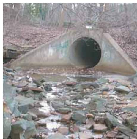
Storm water outfall behind Kings Crossing Center: Storm water from U.S. Route 1 and surrounding parking lots carries automobile toxins into Quander Brook.
