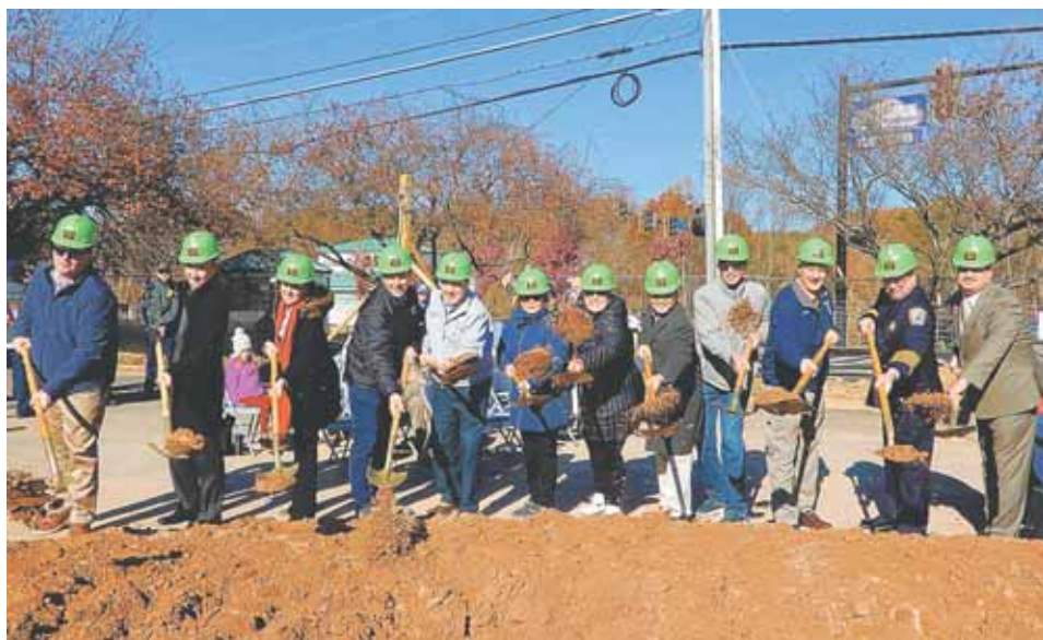
Flinging dirt into the air, current and past Fire Chiefs John O'Neal and Dave Rohr, respectively; City dignitaries; architects and the contractor break ground for Fairfax's new Fire Station 33.
