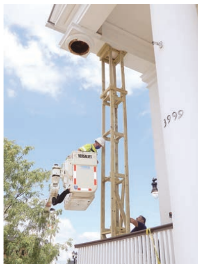
Workmen erecting temporary shoring for Fairfax City's Old Town Hall after a column fell off.
