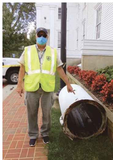
Public Works Director David Summers stands beside a section of the hollow column.
