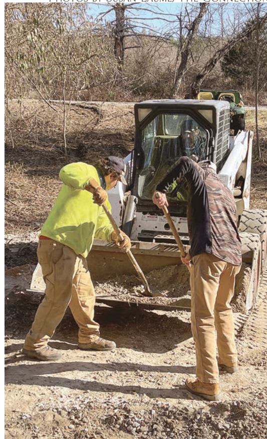
County park maintenance employees Gabe Fetzer and Christian Croke (in cab) work with volunteer Michael Applegate to improve the trail and drain dated from the prison era.
