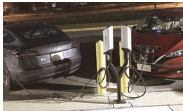
The electric-vehicle charging station outside Fairfax City Hall.
