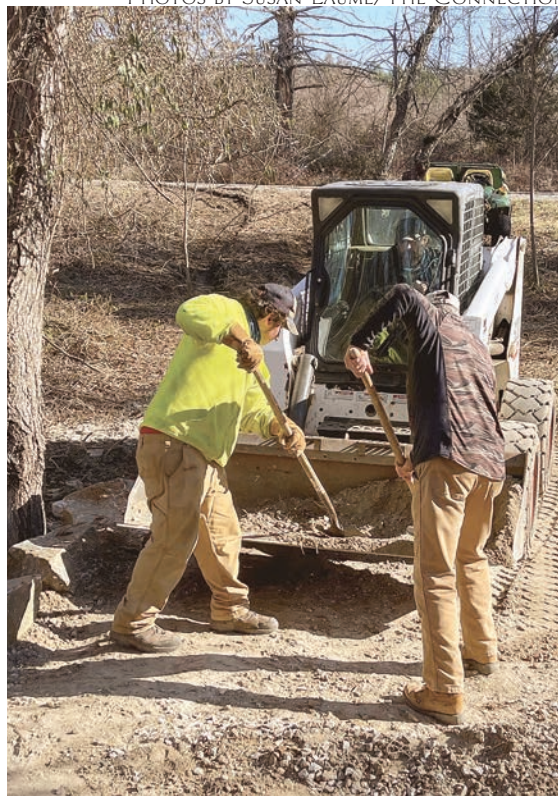
County park maintenance employees Gabe Fetzer and Christian Croke (in cab) work with volunteer Michael Applegate to improve the trail and drain dated from the prison era.
