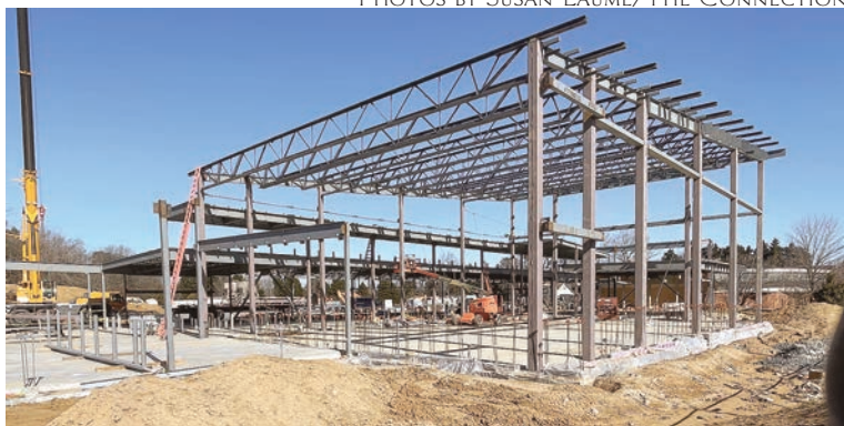
Steel beam outlines of the new Lorton community center dwarf the old library (right rear)
