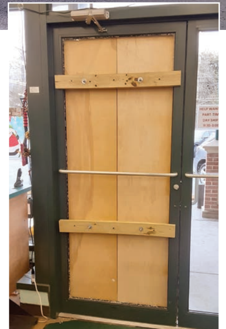
The once glass door at The Variety Store is temporarily covered with plywood. So is the door at River Bend Bistro.
