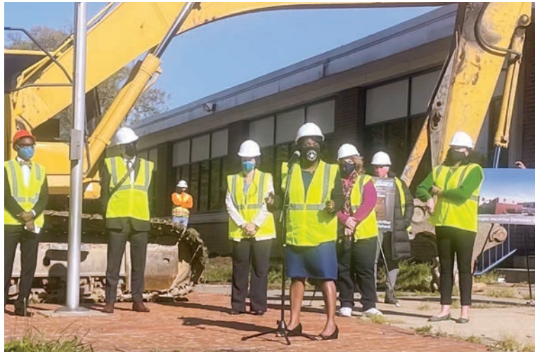
Douglas MacArthur Elementary School principal Penny Hairston speaks on April 26 prior to the beginning of demolition of the 78-year-old school building on Janneys Lane.
