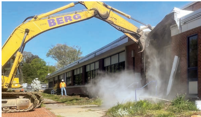
An excavation crane begins demolition at Douglas MacArthur Elementary School April 26 on Janneys Lane.
