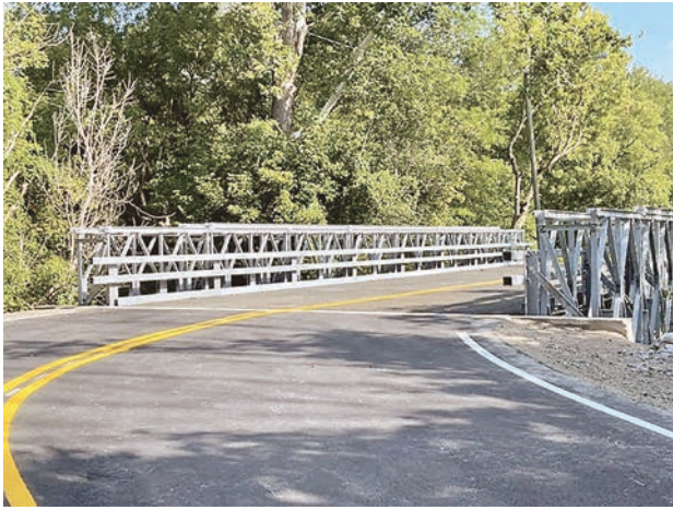
The new temporary span allows re-opening of Old Colchester Road, a link between Pohick and Gunston Roads.
