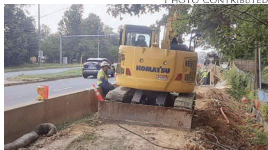
Looking north, the construction crew has had issues with a retaining wall.
