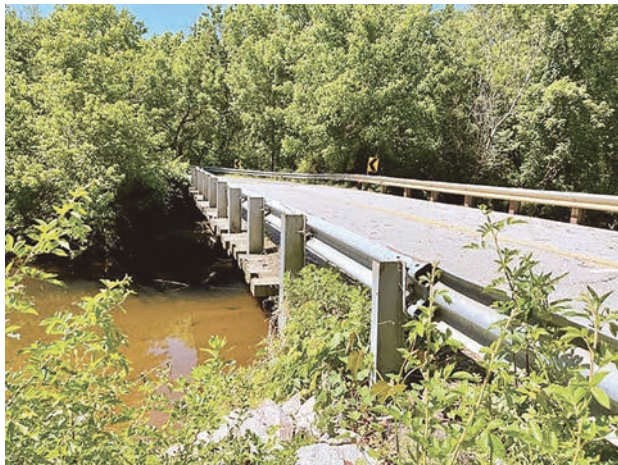
The old bridge, photographed in May, showing signs of corrosion and wood rot, was deemed unsafe for vehicular traffic.
