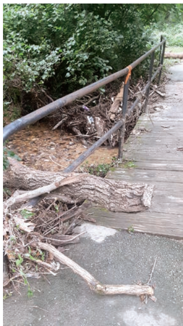
In McCalley Park in the Hollin Hills area, the flooded stream carried debris that impacted a foot bridge.
