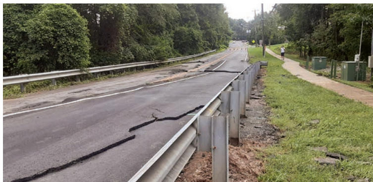
Looking east, the shifted pavement went in the direction of the water.
