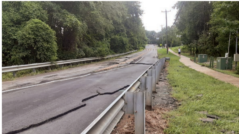
Looking east, the shifted pavement went in the direction of the water.
