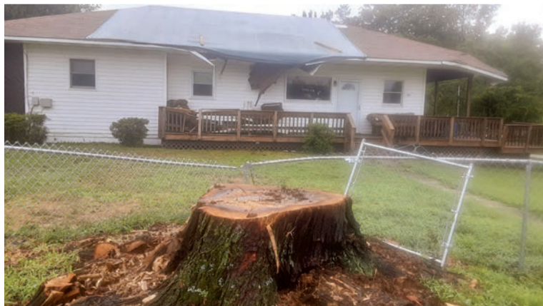
A thunderstorm caused this tree to topple over, damaging this house in Franconia.
