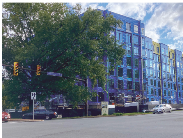
Windows are nearly in as of late September 2021 at the $86 million Lake Anne House Senior House, a new mid-rise planned to serve low-income residents. It is located at 11444 North Shore Drive in Reston and is anticipated to open in 2022, replacing the nearby 50-year old structure.
