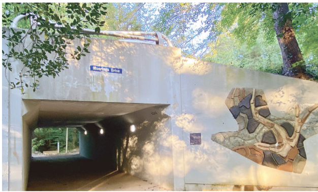
Approximately 24 pedestrian underpasses in Reston improve connectivity throughout the community, many with works of art such as this site-specific nearly 45-year-old bas-relief art mural by Olin Russum at the Moorings Drive Underpass.
