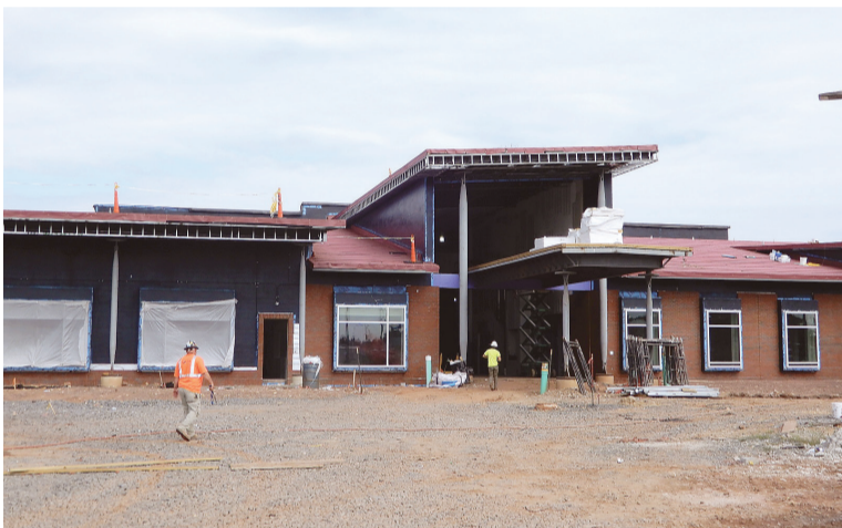
Workmen are busy building the Sully District Community Center near the Udvar-Hazy Center.
