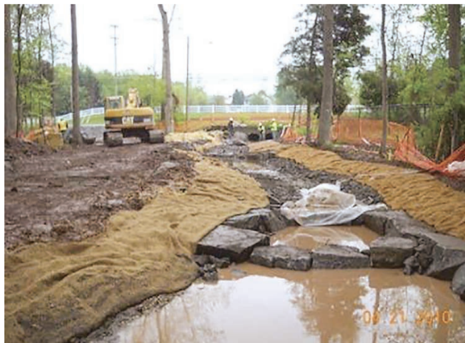
This Fairfax County picture shows what a typical stream restoration entails. Opponents say this is the wrong way to manage local streams.
