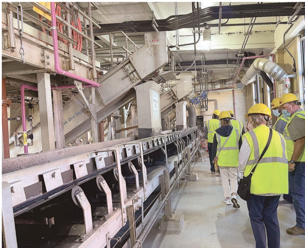
Plant Director Mike McGrath, (white hat) explains one of the primary processes where solid matter and floating materials are separated in covered tanks.
