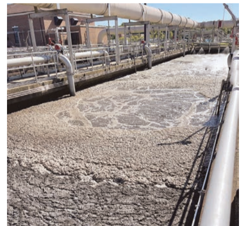
Mid process tanks introduce aeration to stimulate bacteria used to breakdown matter in the wastewater.
