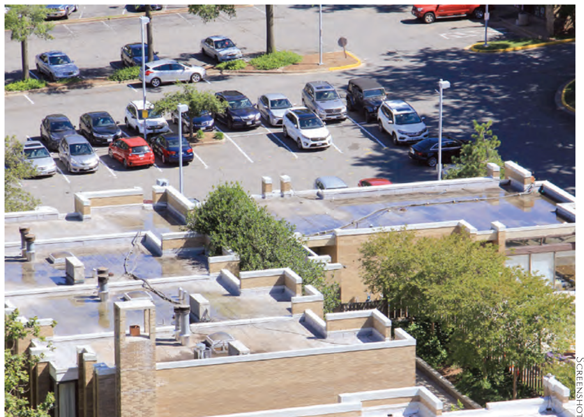
CP-A-10-Chimney House- Ponding water on roof, Roof Replacement $222,670
