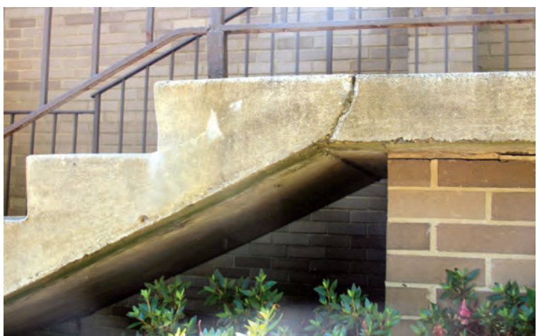
HH-A05 The exterior stair on the South side of Heron House connecting the plaza to the parking lot for Quayside and Heron House residents had signs of deteriorating and spalling of concrete along the underside.
