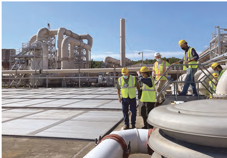
Virginia Master Naturalists observe the Grit Train mechanism that removes materials heavier than water which are hauled to the landfill.
