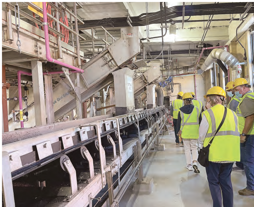
Plant Director Mike McGrath, (white hat) explains one of the primary processes where solid matter and floating materials are separated in covered tanks.
