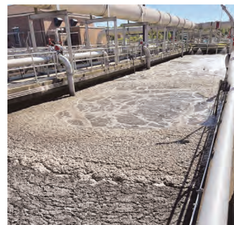
Mid process tanks introduce aeration to stimulate bacteria used to breakdown matter in the wastewater.
