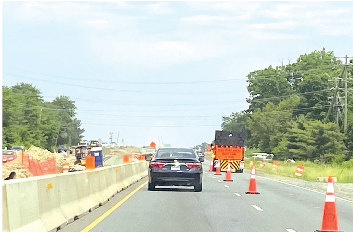
Route 28 southbound traffic traveling in a single lane, while the other lane is closed.
