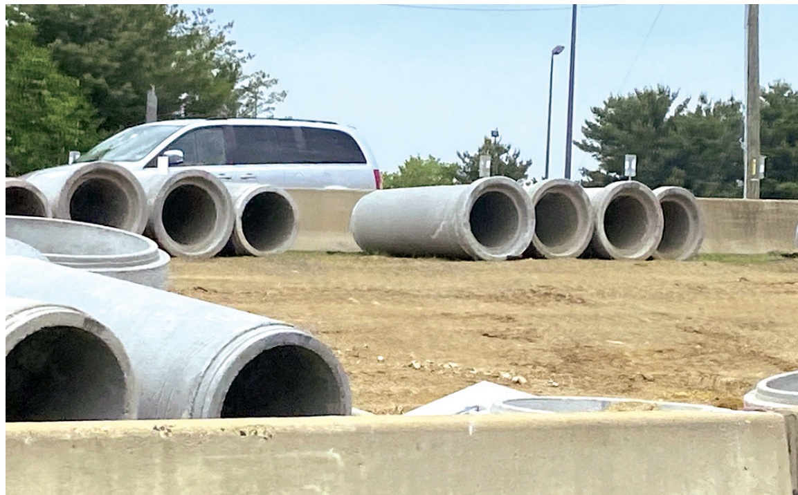
Huge pipes between jersey walls in one section of the median along Route 28.
