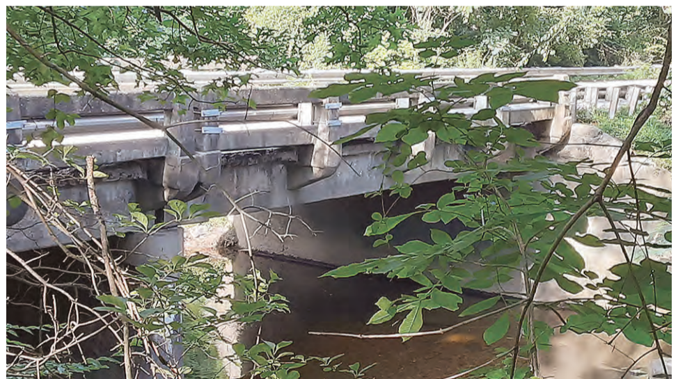
Deteriorating concrete is one reason for the reconstruction.
