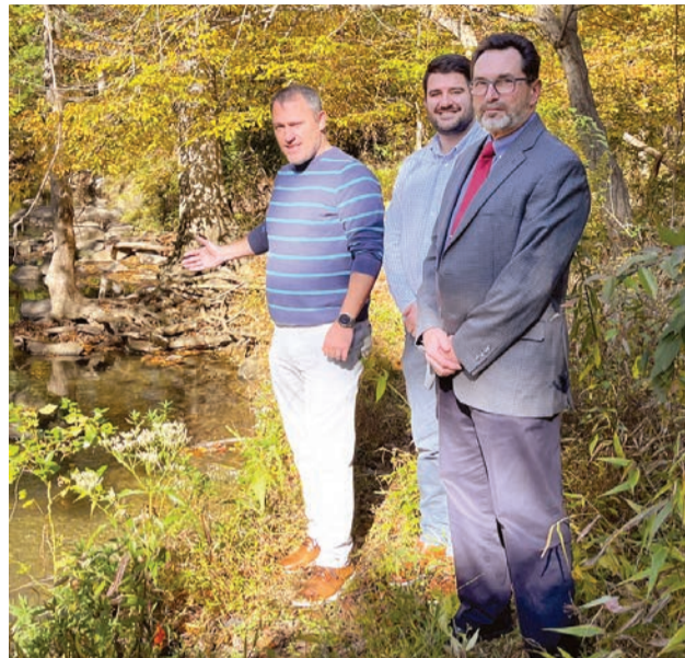
Richard Smith, a senior civil engineer; Lawrence Latour, PE, water resource engineer; and Scott Robinson, director of public works; all with the Town of Herndon, look at the Sugarland Run’s bed and bank erosion.
