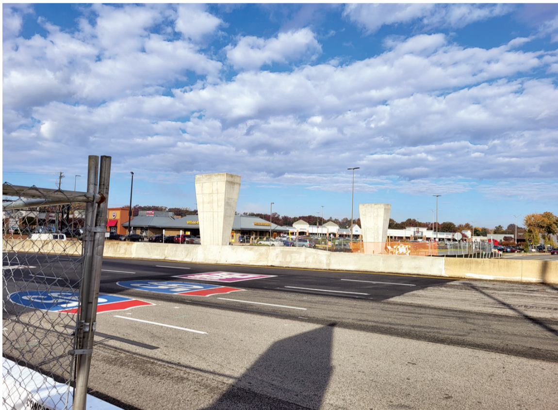
Towers to support the pedestrian bridge that will pass over Old Keene Mill Road.
