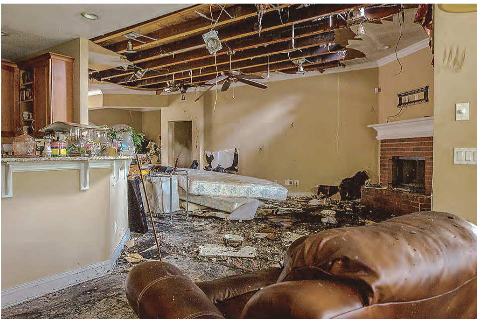
BEFORE: Water damage in Great Falls
