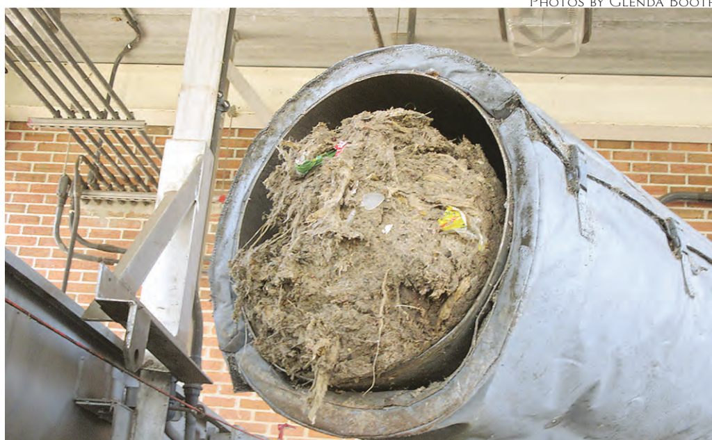
The compacted “leftovers,” solid materials removed from wastewater, like plastics, fabrics and fast food wrappers.
