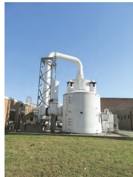
A biotower, odor control technology.
