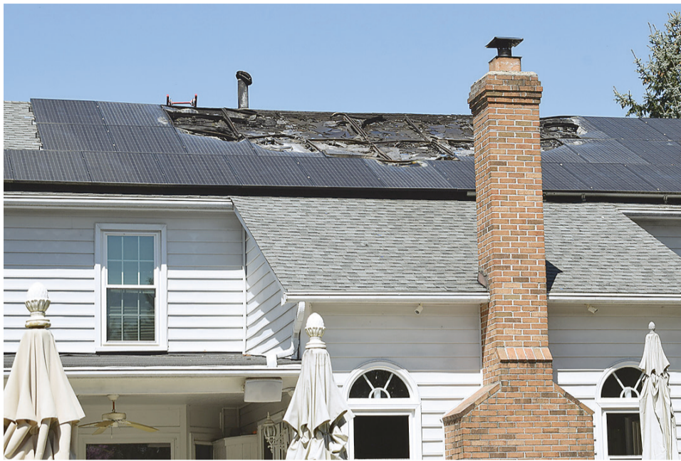
The solar panels on this Centreville house burned.
