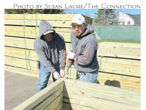
Workers prepare 4 x12 foot raised beds with a group of three making up a rental plot
