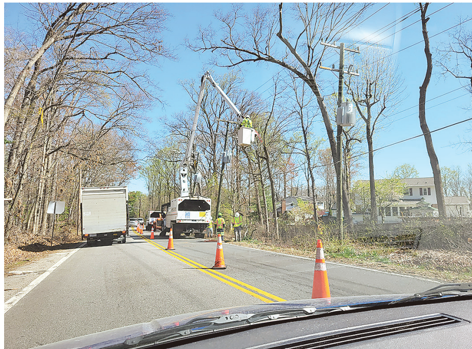
A flagman regulates the flow of traffic during the week here on Rolling Road.
