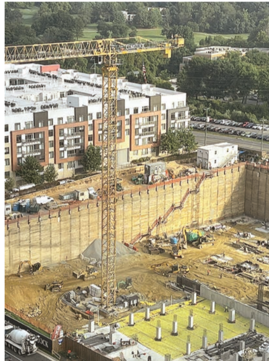
Comstock is continuing to develop the land to the south of Wiehle Metro Reston Station.
