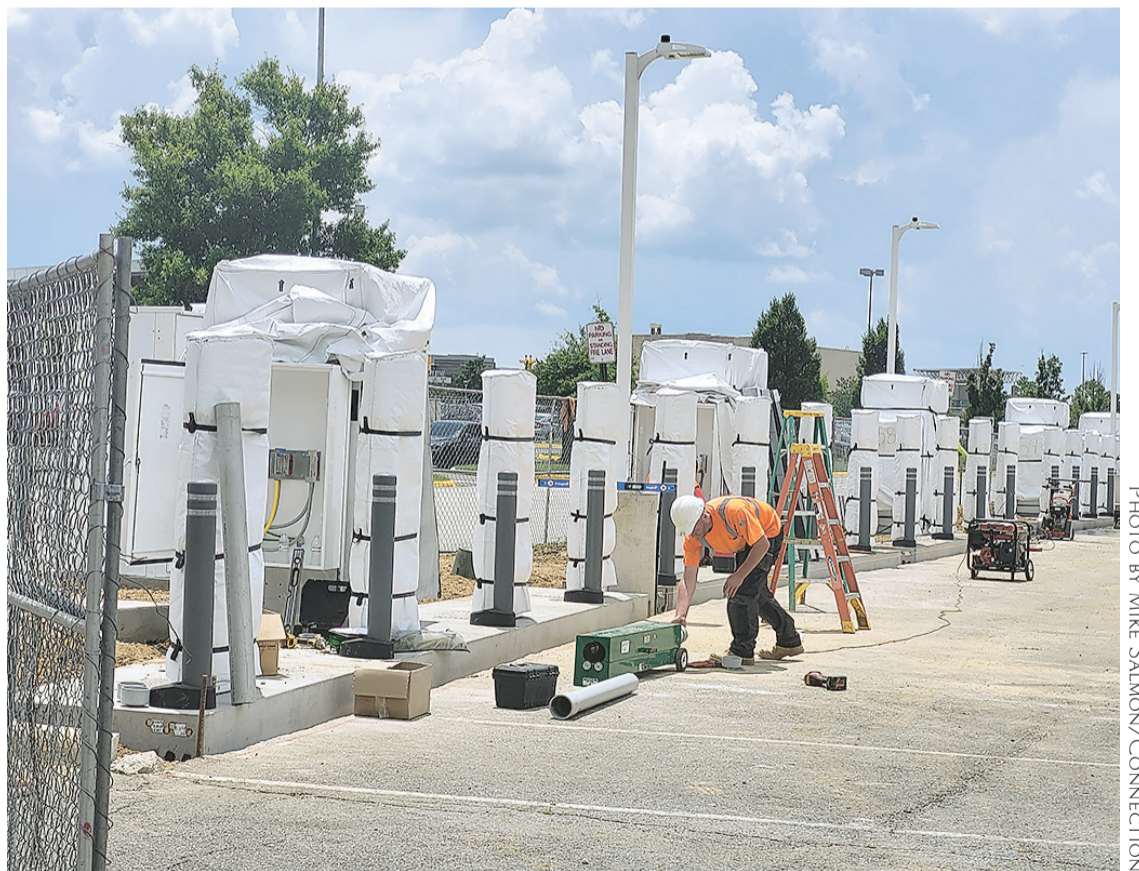
Workers put the final touch on new car charging stations at the Springfield Town Center.
