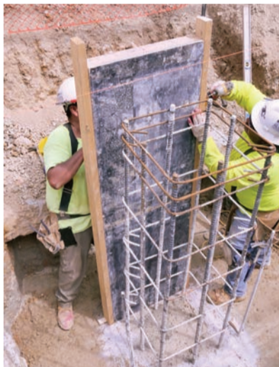
Construction began in June 2022 and in August the workers were digging the building's footings, setting reinforcing bar and pouring the footings.
