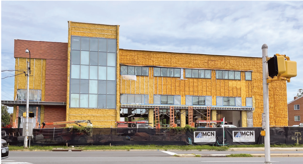
Progress on July 22, 2023 of fire station number 8. The contractor is currently installing brick facade, interior drywall and stairwell guards and laying the gas, water and sewer lines from the building to the street.
